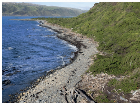
The view south from McGregor's Rock to Shingle Point, showing part of the shore platform damaged by the construction of an unauthorized farm track in 1984. A. June 1972 (Credit: Tony Whitaker, gift of Vivienne Whitaker, 2020, Te Papa CT.066757). B. June 2022 (Credit: Maarten Holl, Te Papa, 206599). The vegetation has recovered naturally from predominantly Coprosma propinqua to taupata ( C. repens ).
